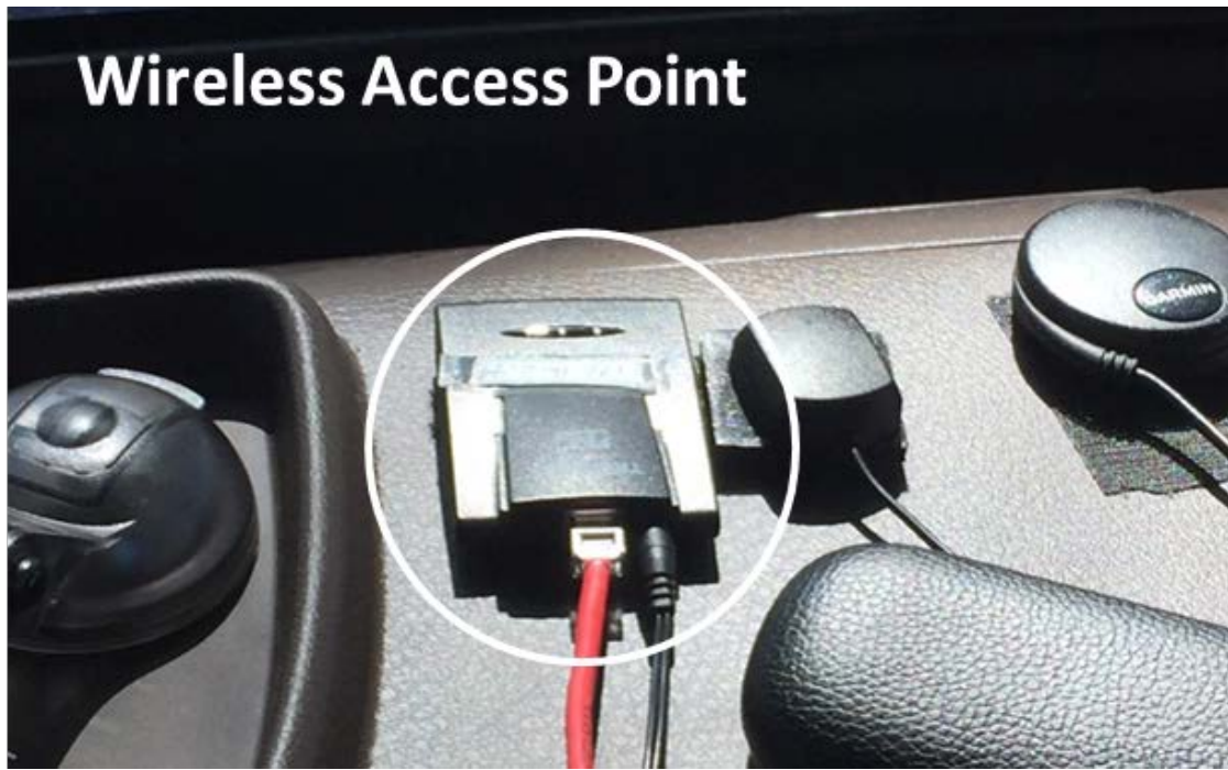
Figure 6. Wireless access point on top of the truck control panel.
