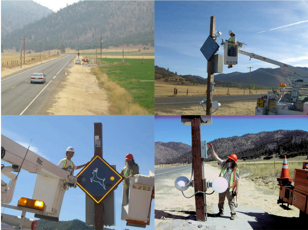
Figure 3: A picture of system installation
