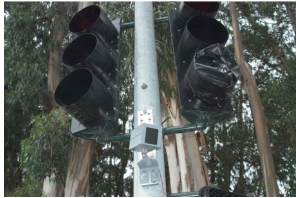
Figure 5.6 Pedestrian Detection Sensor mounted on the Signal Pole
