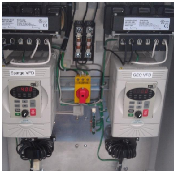
Figure 2.4. VFDs used to control the pumping rate of the culture through the PBR tubes. Two independent prototype systems, each requiring a VFD, were constructed during the OMEGA project.
