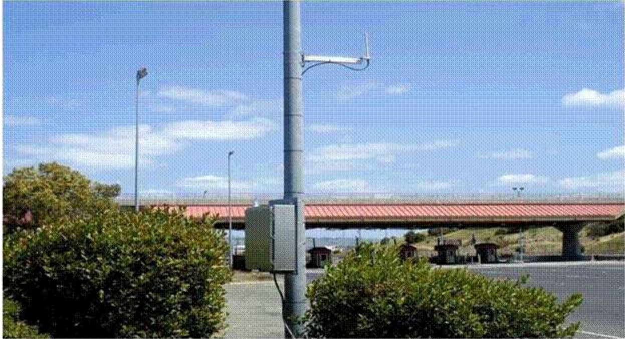
Figure 4-8: DSRC communication installation for VII testbed [ www.vii.path.berkeley.edu ]
